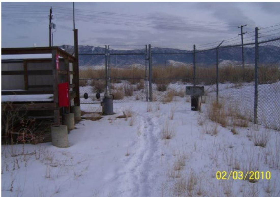
Figure 4-2. West Camp pump station 1997–2011.
