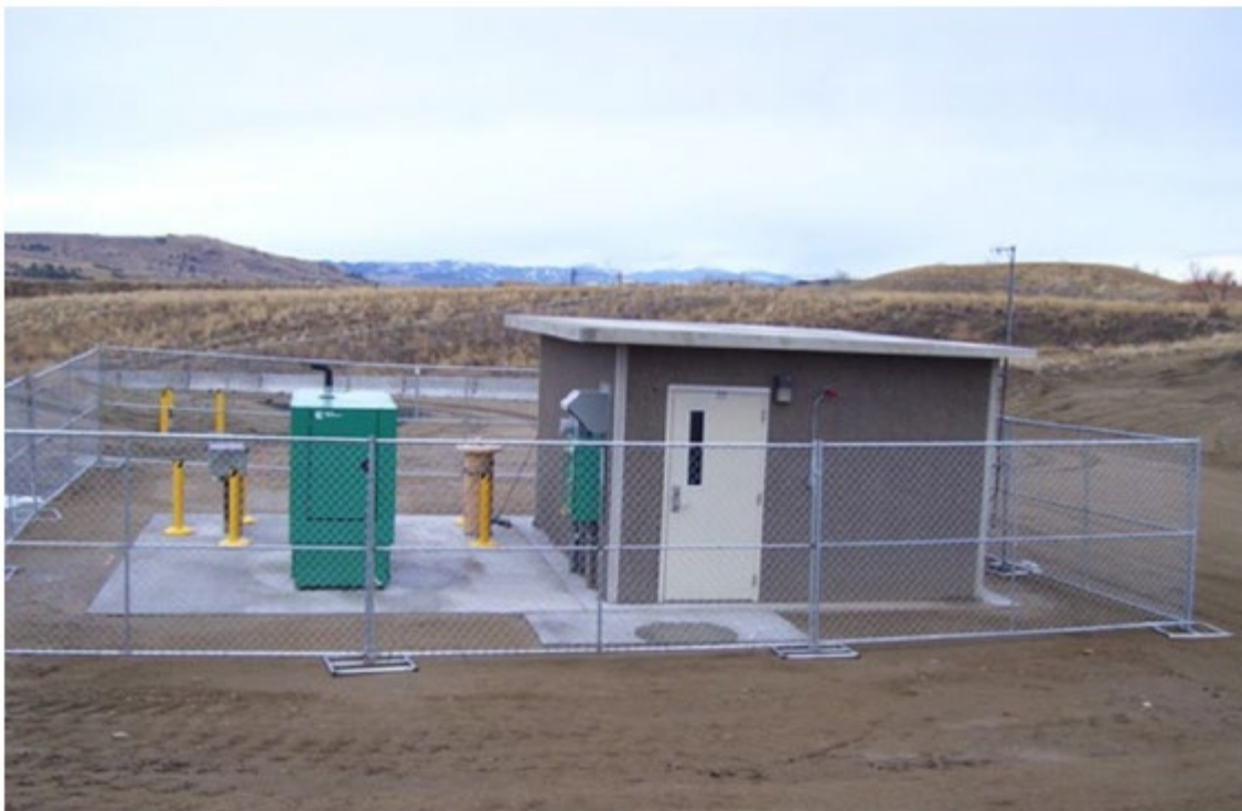
Figure 4-5. West Camp pump station upon completion in 2011.
